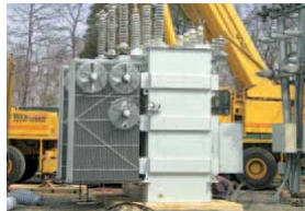
A crane is used to install a large, 30 MVA transformer at the Evergreen Substation.
