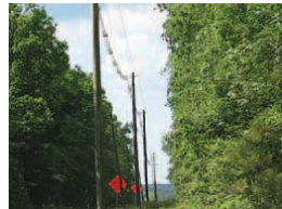
A Hendrix spacer cable is installed along this heavily wooded stretch of Bull Run Post Office Road. The durable cable is engineered to fit in tight spaces and customers can expect more of it in coming years.
