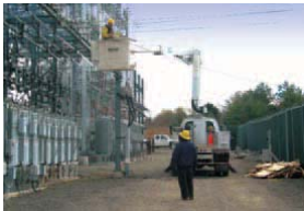
In preparation for upgrades at Cub Run Substation, Electrician 1st class Mark DeChristopher begins the arduous task of dismantling the old circuit bus.
