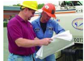
Quality assurance inspector Kevin Bowling (left) reviews site plans with a contractor to ensure NOVEC specifications are met.
