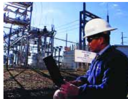
Substation engineer Arnel Majillo collects real-time diagnostic information from a NOVEC substation.
