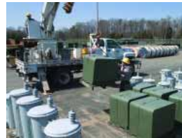
Maintaining the appropriate inventory level is key to meeting the demands of rapid construction.
