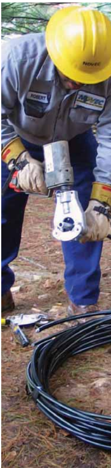
NOVEC line technician Robert Jackson prepares to splice a cable during an underground fault repair.
