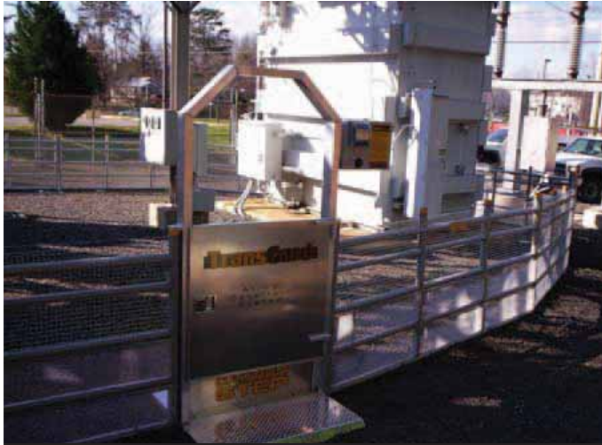
NOVEC uses special fences in substations with a prevalent squirrel problem, such as at Stonewall, Sudley, Ballsford and Cardinal substations. The inner fence, pictured here, is energized to give squirrels and other animals such as snakes and raccoons a mild shock to deter them from climbing any further and potentially causing an outage at the substation.
